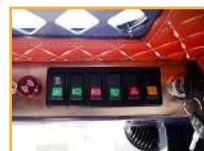
PANEL DE CONTROL
